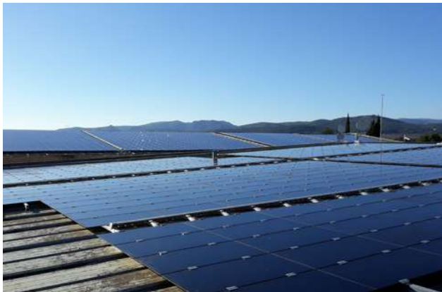
Photovoltaic system in the Penedès winery
