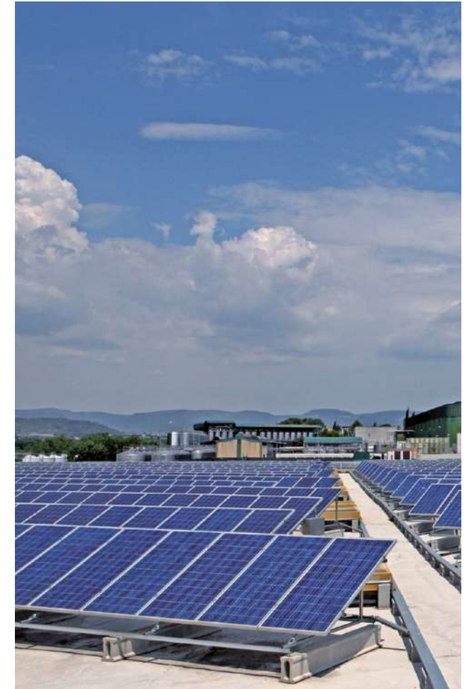
Photovoltaic system in the Pacs del Penedès winery
